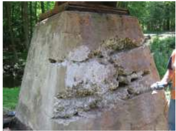
Fig. 4.1.4a—Trestle of the railway bridge before repair.
