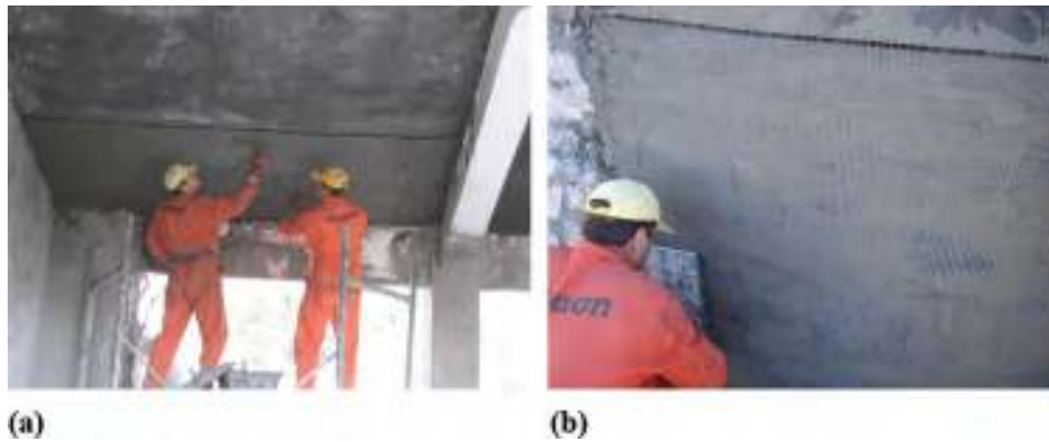
Fig. 4.2.2—School building strengthening of: (a) concrete slabs; and (b) stone masonry walls.
