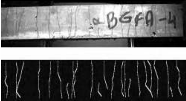
Fig. 3.2.1b—Distributed cracking in AR glass-FRCM (width = 1 in. [25 mm]).
