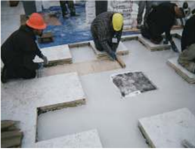
Fig. 4.1.1—Installation of FRCM on roof slab around area where slab opening will be cut for duct passage.
